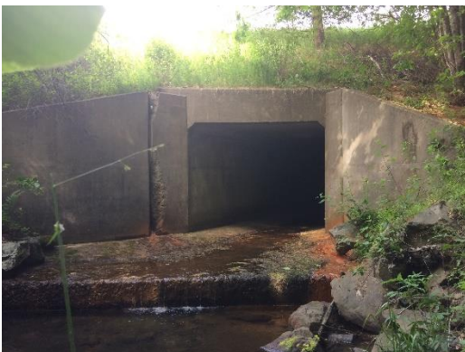
Figure 29. Example of a V bottom box culvert , with “dry concrete” movement surfaces along culvert walls. Site I91-17-2, Putney.
